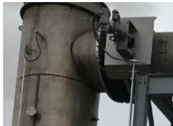
Figure 3- A hot gas isolation valve provides a simple and effective automated protection of downstream equipment, allowing the landfill gas flare to run continuously and independently from the leachate management process.
