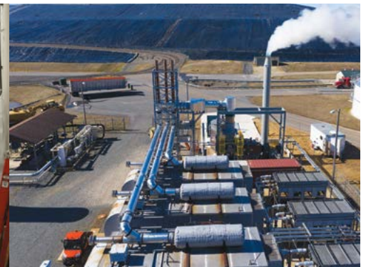
Figure 3: Hot generator exhaust gas is ducted together to provide thermal energy for evaporation in the Heartland Concentrator™.
