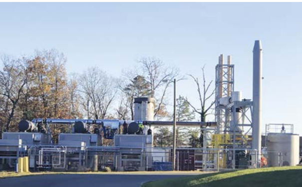
Figure 1: Profile view of the Heartland ROVAP™ Reverse Osmosis Concentrate Evaporation Facility.
